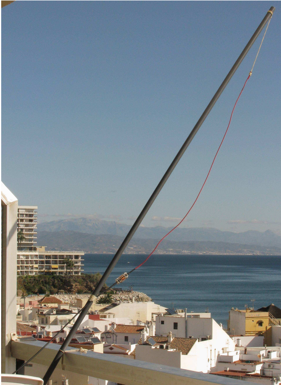
Figure 13: Photo of the antenna installed on a front side Balcony of the Nucleo Cristal building (the A building), in La Carihuela (Torremolinos-Málaga-Spain).
